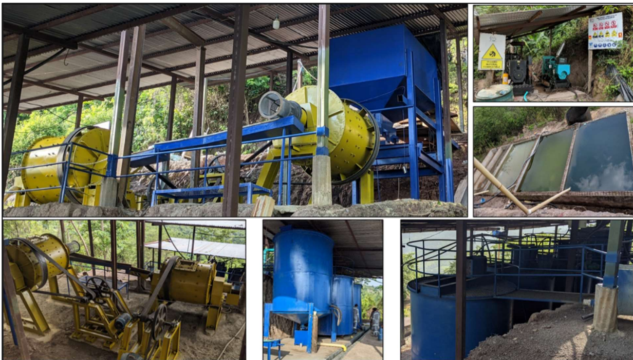
Image 3: Pilot plant equipment on-site at the Santa Barbara Gold Project
